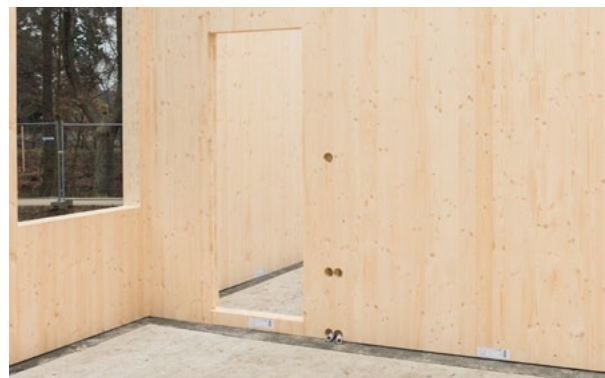
Preparation for electrical wiring inside the panels across the entire height of the walls.
