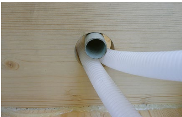
Gooseneck pipes (ELEMENT).
