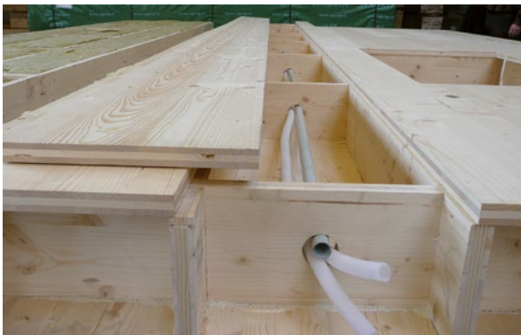
Longitudinal cut-out in the upper board, unglued for wiring and piping installations.
